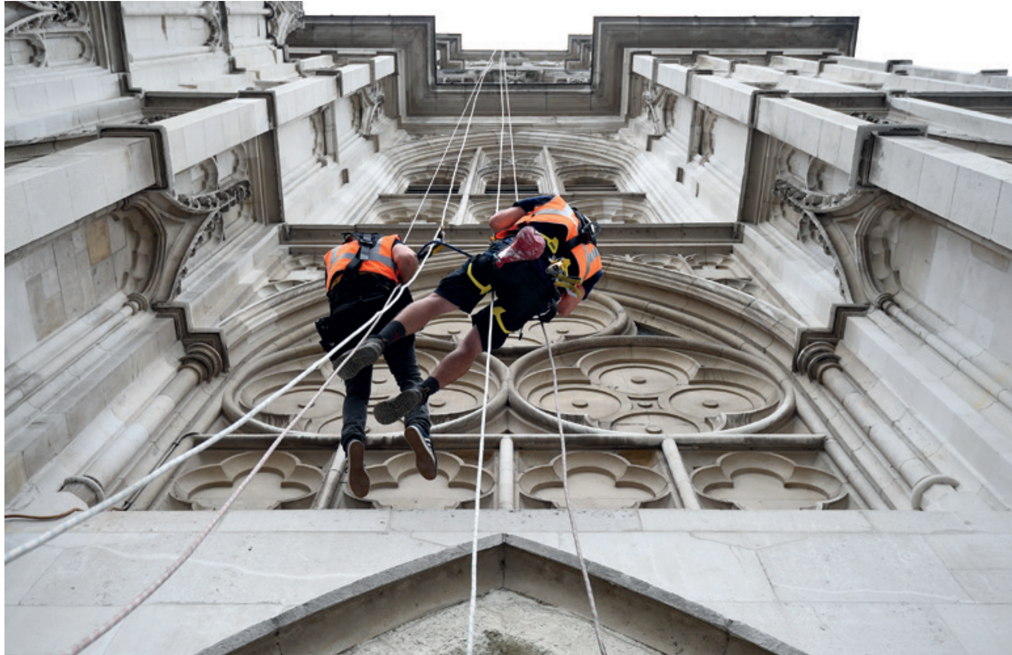
Despite coronavirus, essential building maintenance work continued at the Abbey – including abseilers checking the masonry of the west towers.
